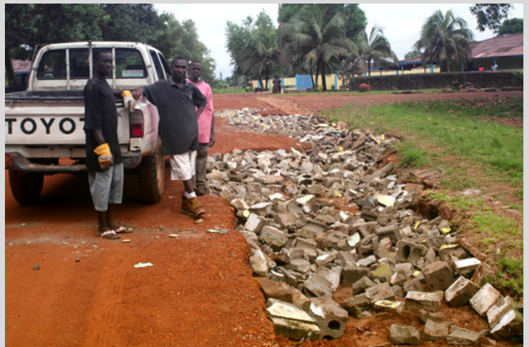
There is much to do in and around the clinic. TDC helped repair the road in front of the clinic, badly eroded by rainy season, with bricks from the staff house and clinic demolition. Destruction is good for something!
